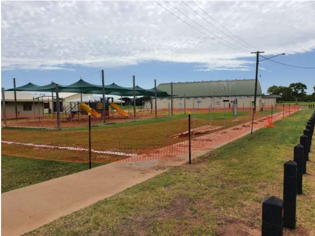
Photo: Installing fence posts and concrete footings at the Kath Alexander Park.
