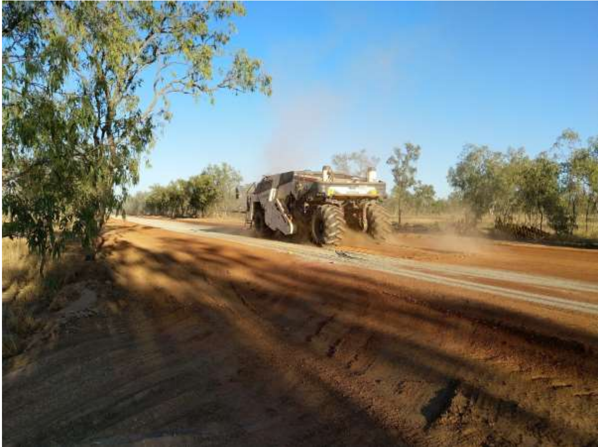
Photo: Stabiliser dry mixing cement powder into the base pavement on 89B.
