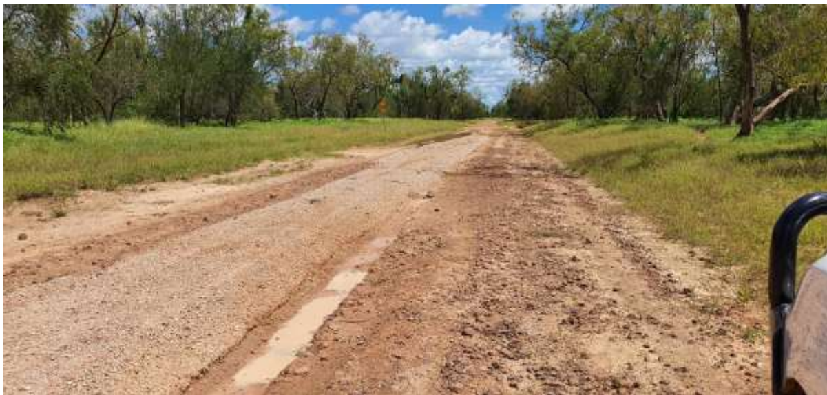
Photo: Gravel Washouts on 89B
