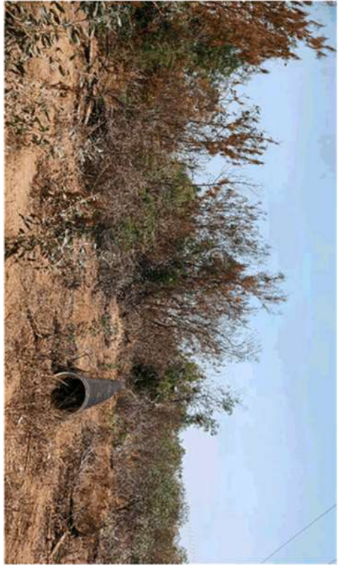
PMP 6.2 – After (previously impenetrable Senna alata , Bellyache bush, Neem tree and Rubber vine)
