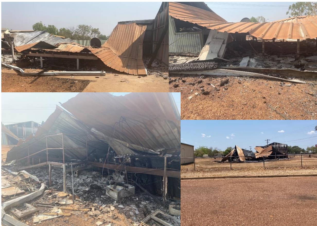
Figure 5 – After the fire, showing damage caused to the House
