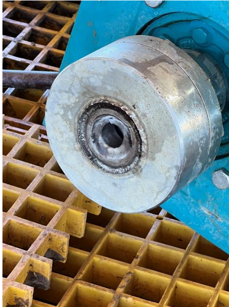
Photo: Normanton WTP Clarifier 2 Mixer Shaft failure
